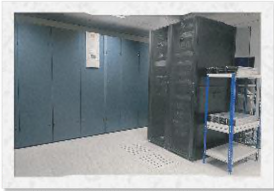
DATACENTER HQ ML&C Rwp
